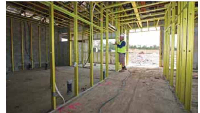
Assistant Project Manager Brett O'Brien inspects construction of the dog adoption pens inside the main building.
